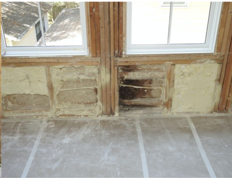
Figure 24.2 - Sheathing moisture damage
