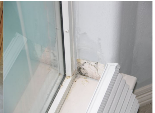
Figure 24.3 - Mold at windowsill
