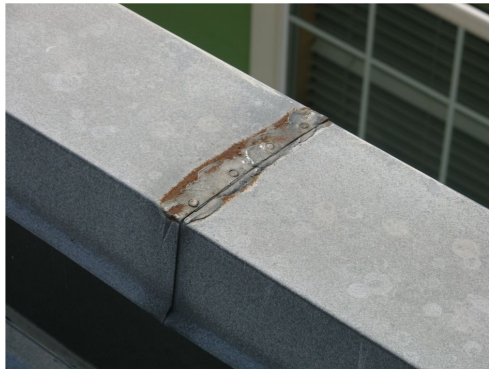
Figure 27.2 - Cap flashing separations
