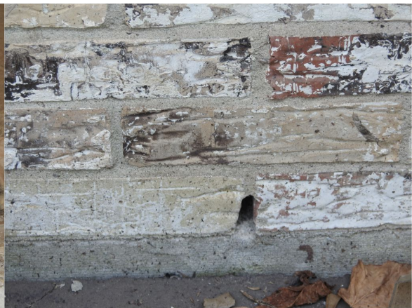
Figure 23.4 - Plugged weep hole
