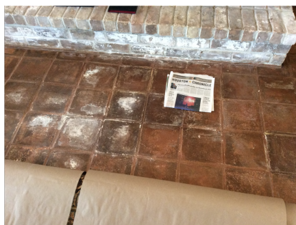
Figure 26.2 - Moisture from damaged vapor barrier
