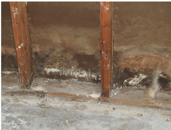
Figure 23.3 - Sheathing moisture damage
