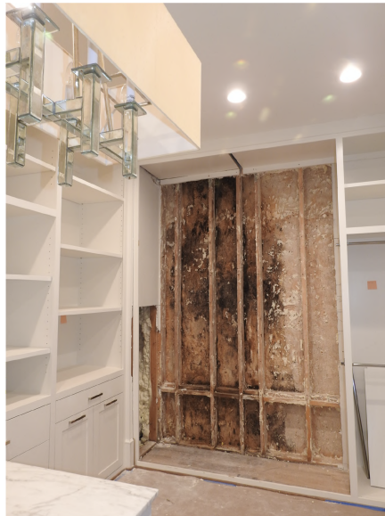
Figure 26.1 - Scupper leakage damage
