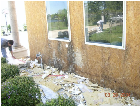
Figure 24.1 - Sheathing moisture damage
